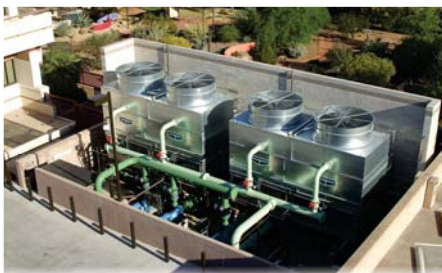
City of Peoria Cooling Towers
