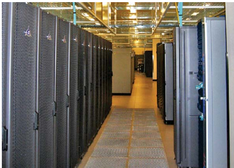
Client Data Center
