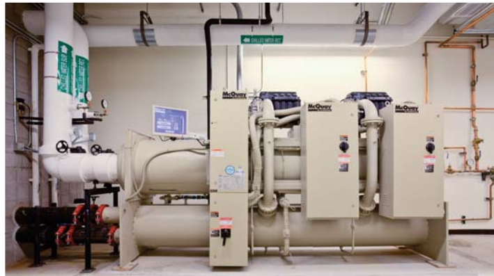
Climatec Headquarters Chiller Plant
