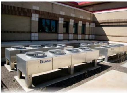
Peoria IT Building Cooling Fans
