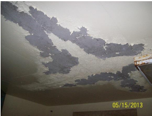
Spalling and deteriorated concrete slab
